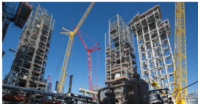
Photo: Construction of the polyethylene units at Old Ocean, Texas, is progressing.
